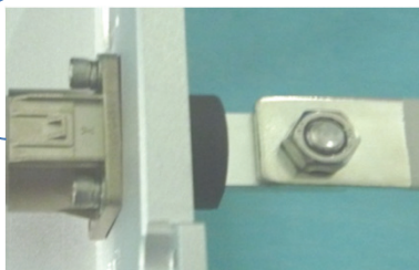
e、 取出安装辅助治具后完成安装 Complete installation after taking out the fixture .
